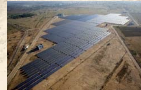
A 5 MW grid-connected solar power plant at Khimsar village, Jodhpur, Rajasthan.
